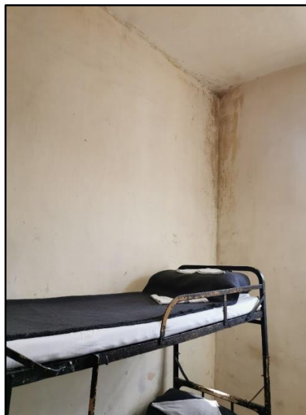
Traces of leaking
