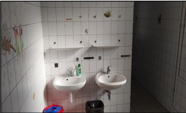
Plumbing unit of the mother and child unit
